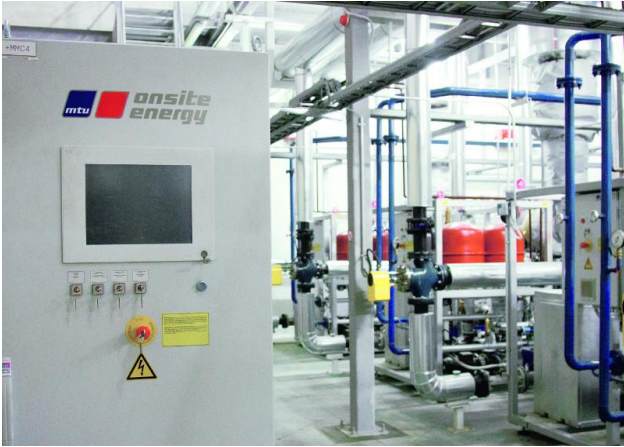
FIGURE 9: CURTIS POWER SOLUTIONS: CHP
