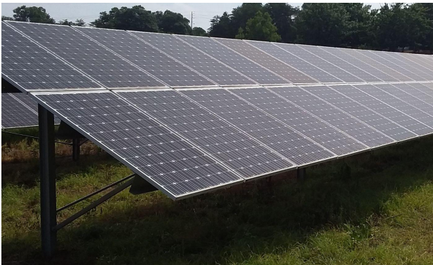
FIGURE 4: ON-SITE POWER GENERATION
