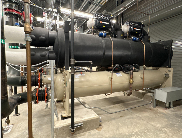
FIGURE 2: DAIKIN WATER-COOLED CHILLER
